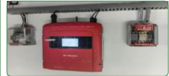
Solar Inverter System
