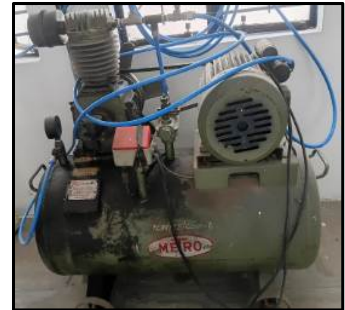
Compressed Air Energy Storage
