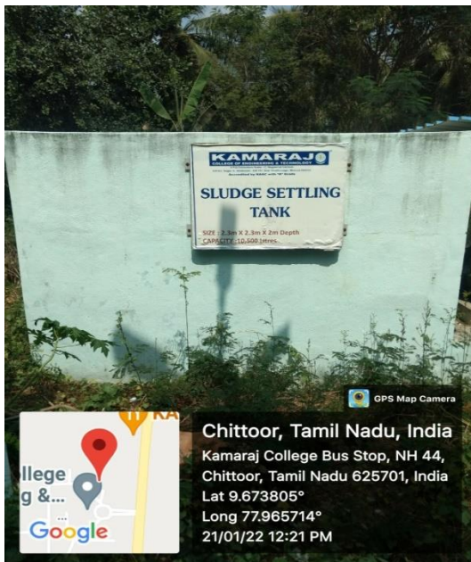
Fig. 7.1.4.10 – STP – Sludge Settling Tank
