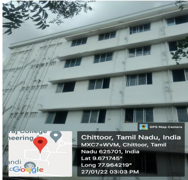
Fig. 7.1.4.12- Drinking water distribution pipe line behind E-block
