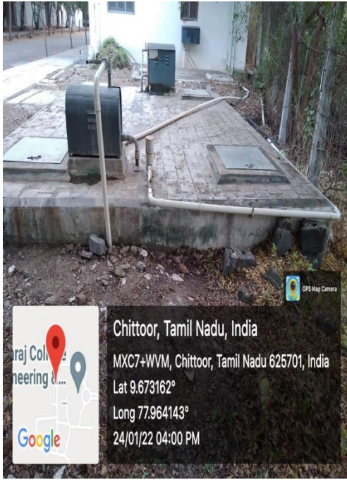
Fig. 7.1.4.1- Rainwater sumps at Site Office
