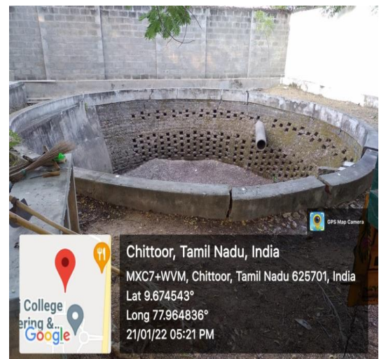
Fig. 7.1.4.4- Rain water pond harvesting sump at girls hostel
