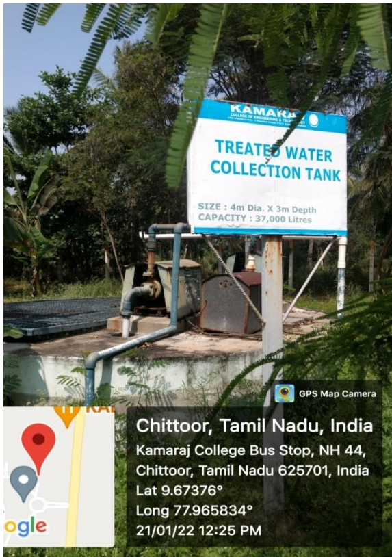
Fig. 7.1.4.8 – STP – Treated water collection tank
