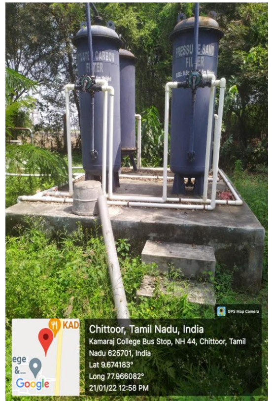
Fig. 7.1.4.9 – STP – Activated Carbon and Sand filters
