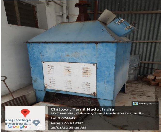
Fig.7.1.3.4-Sanitary pad disposal unit in ladies hostel
