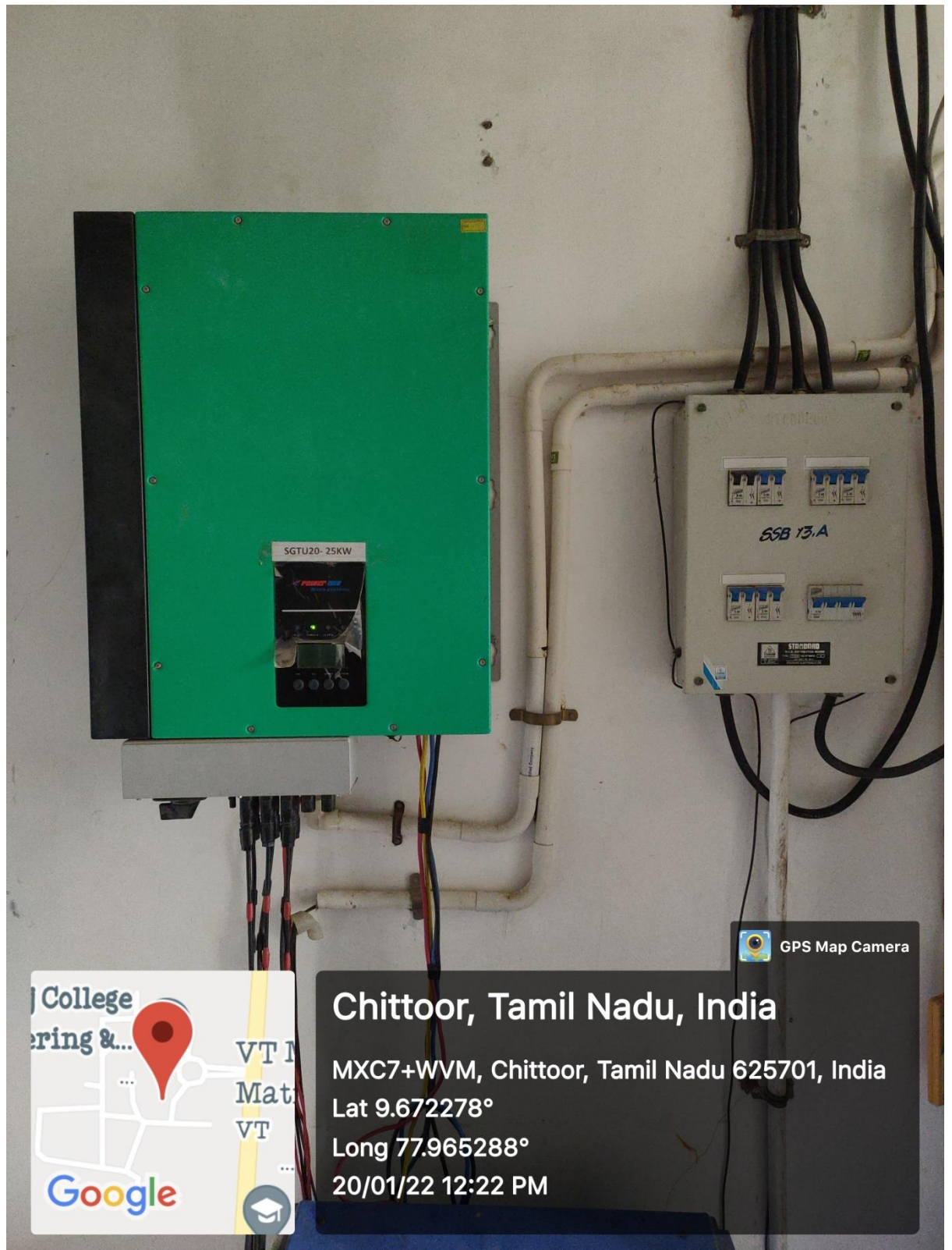
Fig: 7.1.2.2.b Grid Connected Solar PV Inverter in B Block
