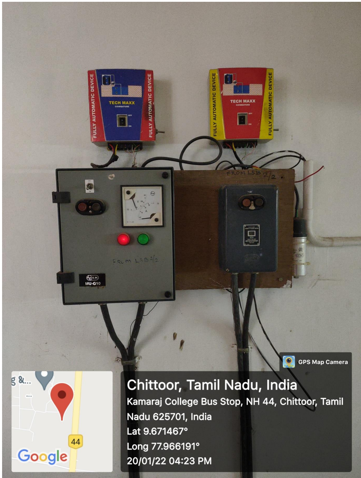
Fig: 7.1.2.6.a .Starter for Automatic Water Level Controller
