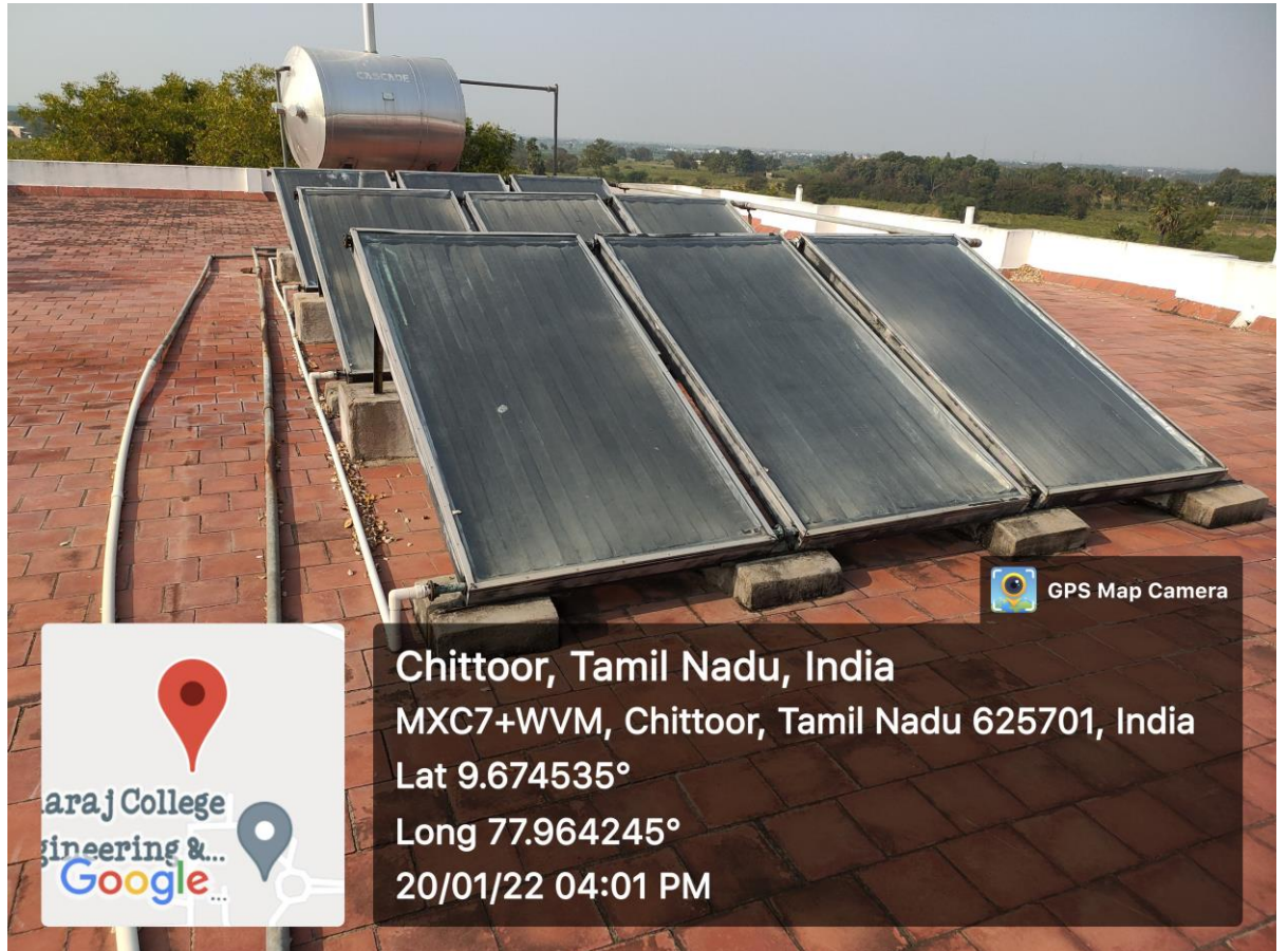
Fig: 7.1.2.2.c Solar Water Heaters in Girls Hostel
